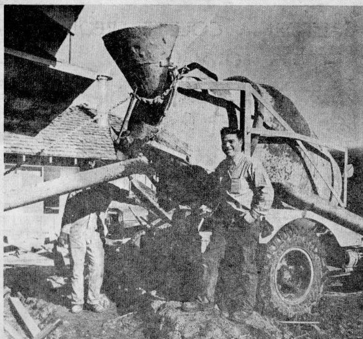
The development and building program of Christmas Valley goes on 7 days a week. These workmen are putting in a concrete foundation for still another building. Buildings are going up so fast, that the landscape changes almost weekly. And the M. Penn Phillips Company promises there'll be no letup in the building and development program to make the Valley the ideal place to live and play.
